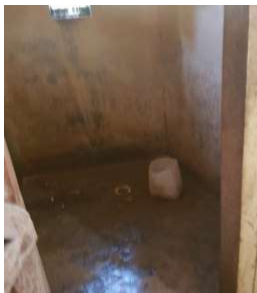
Very poor sanitary facility at the Prisons
