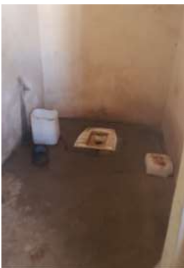
Poor sanitary facilities
